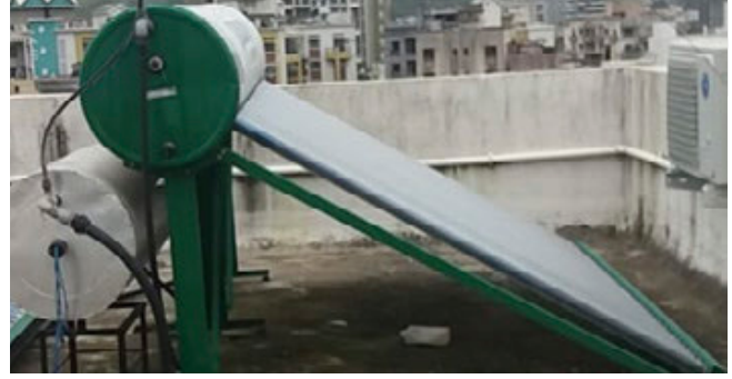
500 LPD Solar Water Heater
